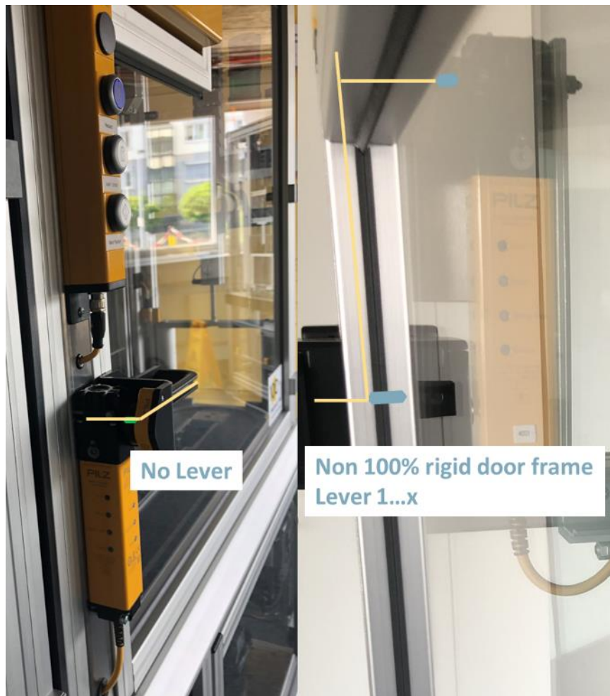
Figure 8: Leverage on a guard locking device on gates
