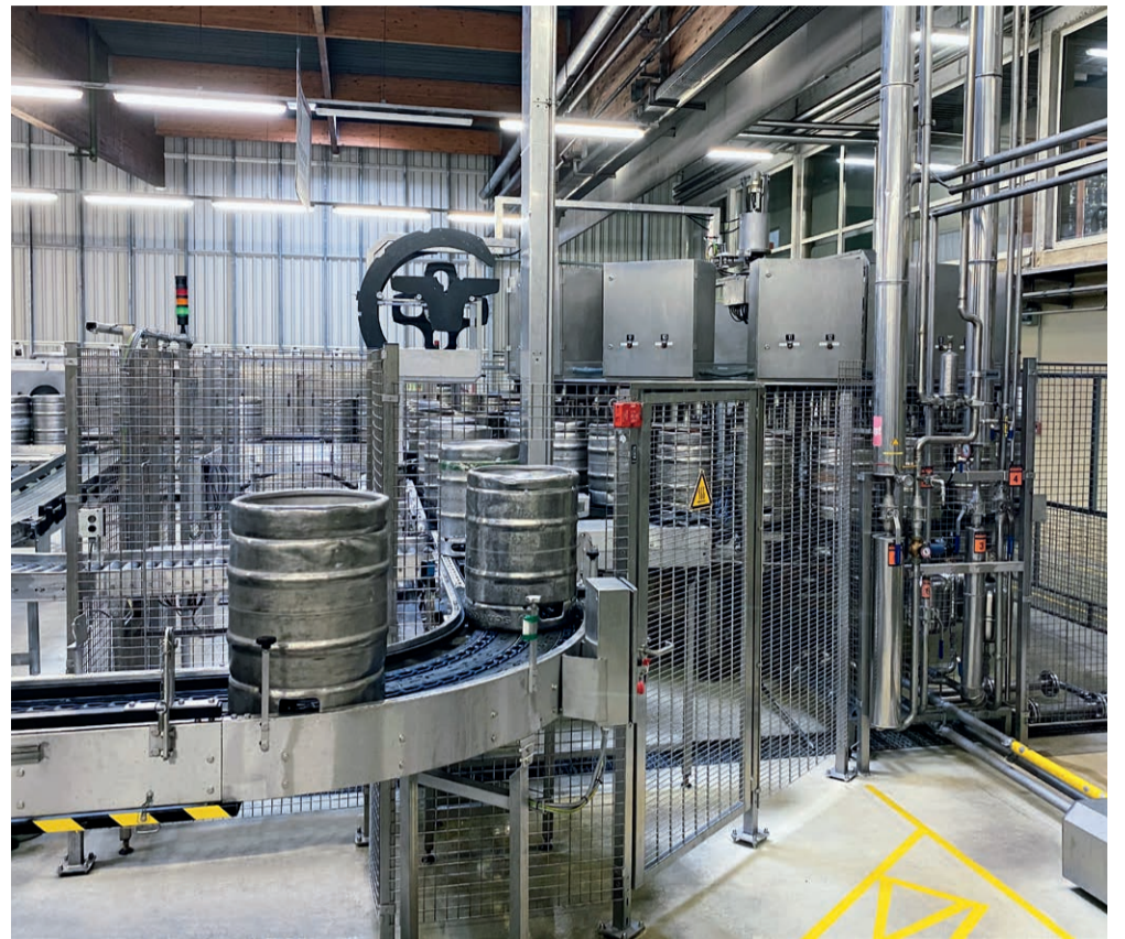
As part of a controller retrofit, one of the tasks for safety experts was to re-assess and validate options for intervention on the machine.
